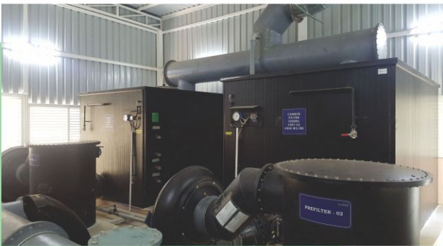
Activated Carbon Filter
