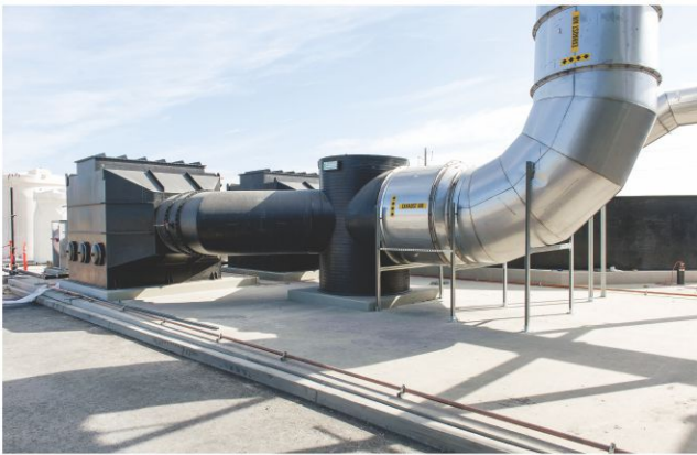
FRP Ducts & Pipes
